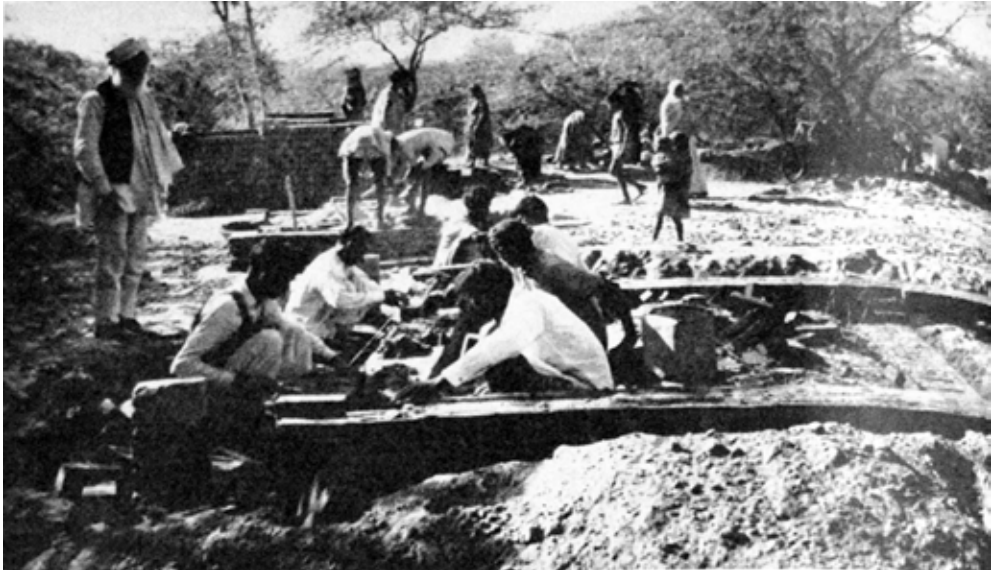
Figure 4. Local villagers demonstrating construction of rural houses by the self-help method. Source: United Nation's Bulletin, March 1, 16(5), pp. 186-191, p. 186, © UN.
